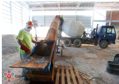
Fibre Integration At Site
