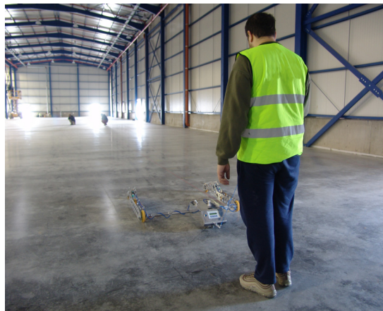
Face Consultants survey the floor according to DIN 15185 before the racking installation
