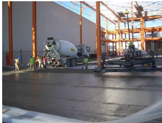
Construction of second slab in progress. Concrete truck and Laser Screed working alongside each other. Smooth output ensures highest quality is achieved with no delays.
