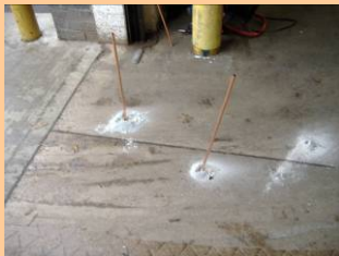
Injection ports and drill holes for slab stabilisation grouting to the Goods In area of a warehouse
