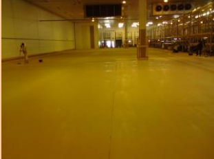
1st coat application of Solvent Free Epoxy High Build Coating to the Milk Store area
