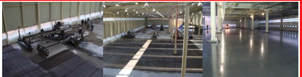
From left: Laser Scream & Topping Spreader in action; floor construction; Completed floor.
