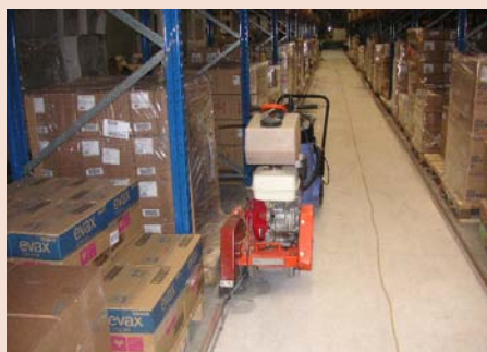
Completed laser ground aisle at HEFAME
